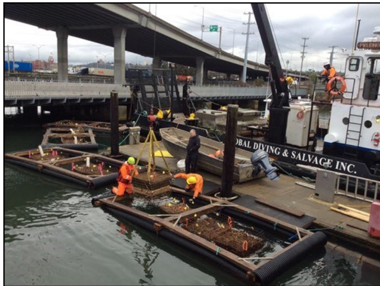
Installing the floating wetlands within the biobarges before relocating them to their future sites (credit: University of Washington Green Futures Lab)
